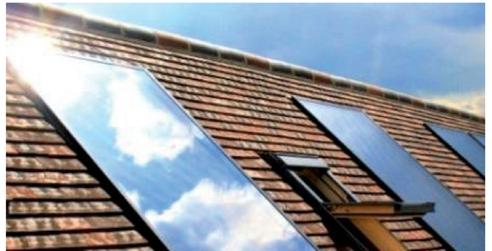
PV SOLAR PANELS
